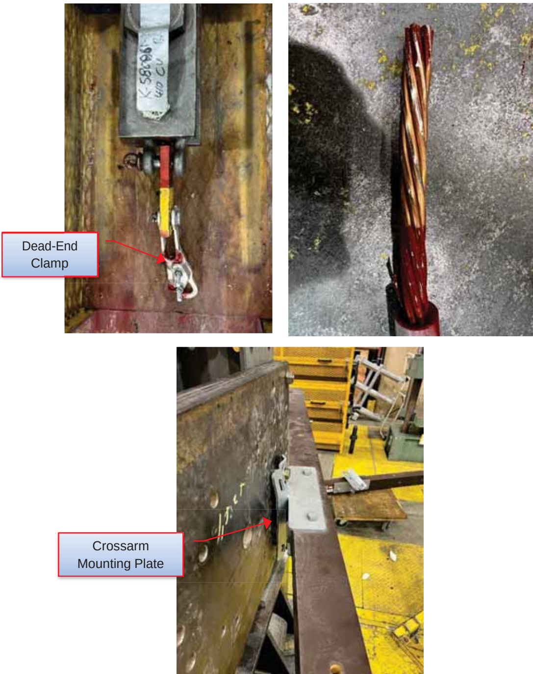
Figure 6-16: Sample 3.3 – Failure Location
