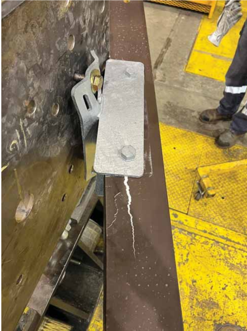
Figure 6-17: Sample 4.1 – Failure Location
