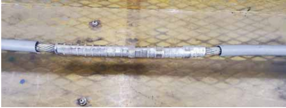
Figure 3-4: [REDACTED] Installed on 22 kV 397.5 kcmil, 19 strands AAC
