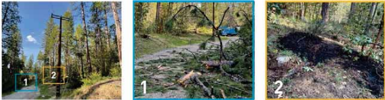
Figure 3: PG&E Covered Conductor Effectiveness – Example 2
