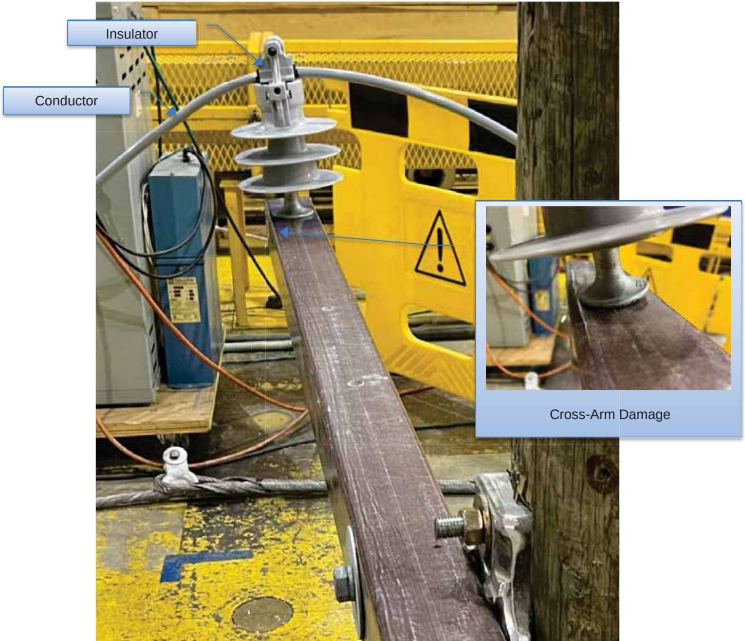
Figure 6-21: Sample 3.4.1 – Insulator and Cross-arm Condition after Test
