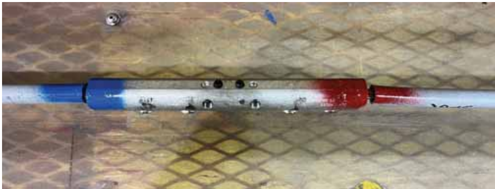
Figure 3-5: [REDACTED] Installed on 15 kV 1/0 AWG, 6/1 ACSR
