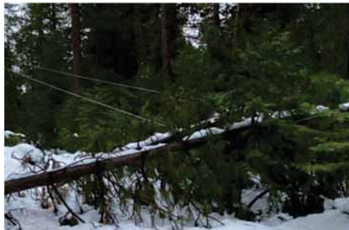
Figure 4: PG&E Covered Conductor Effectiveness – Example 3
