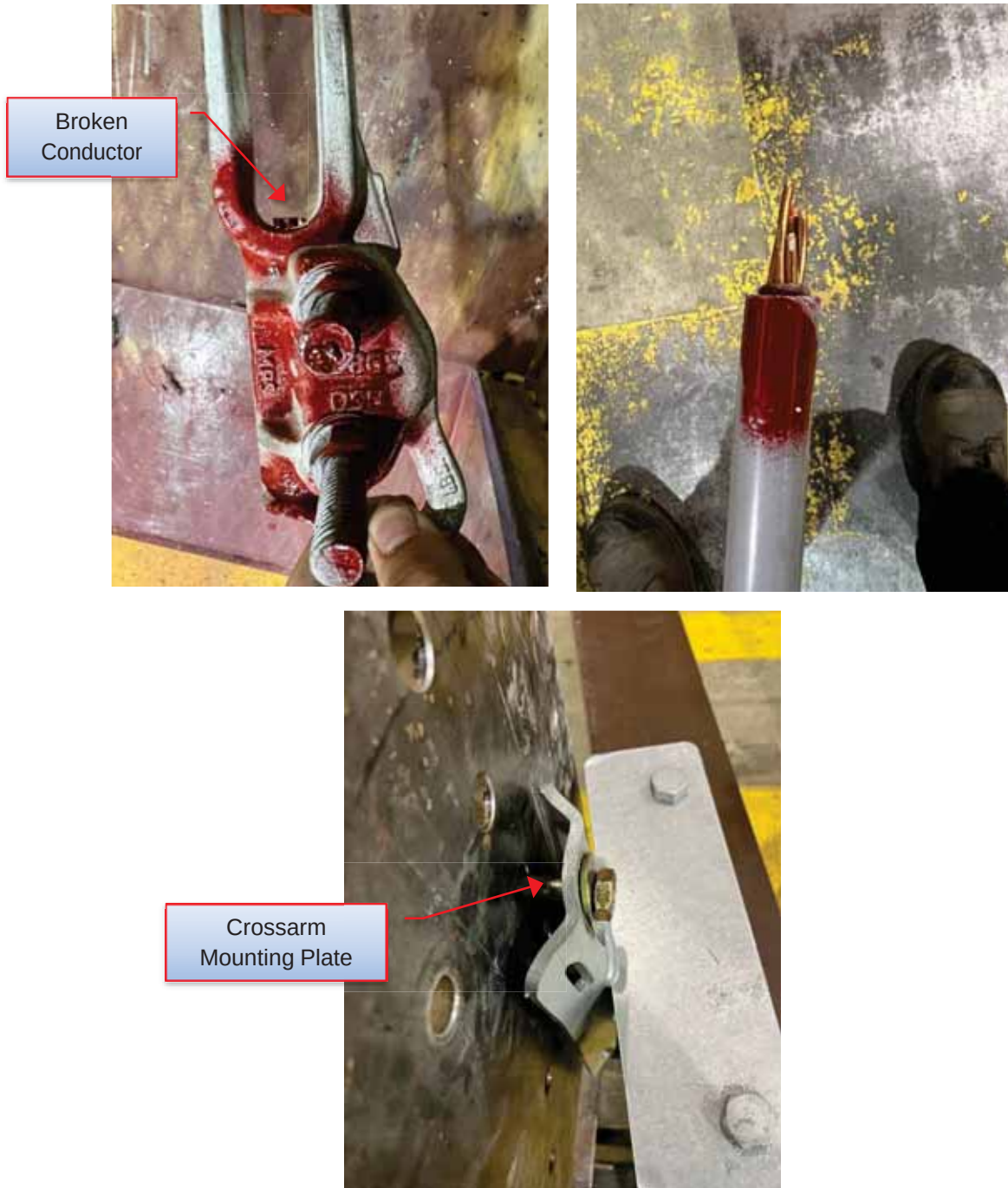
Figure 6-8: Sample 1.1 – Failure Location
