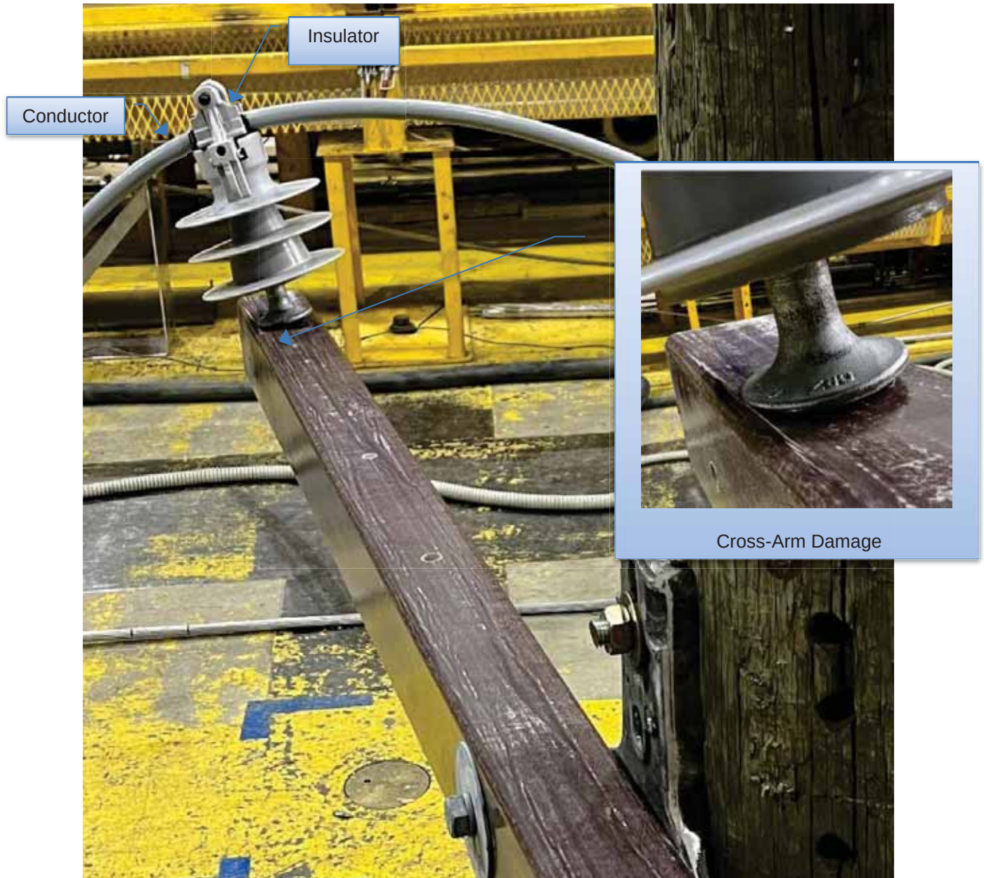
Figure 6-13: Sample 3.2.1 – Insulator and Cross-arm Condition after Test
