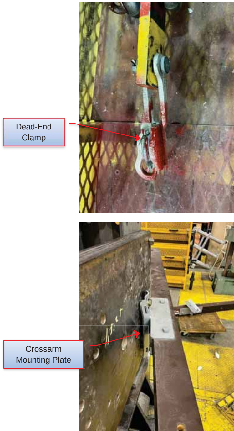
Figure 6-15: Sample 3.2 – Failure Location
