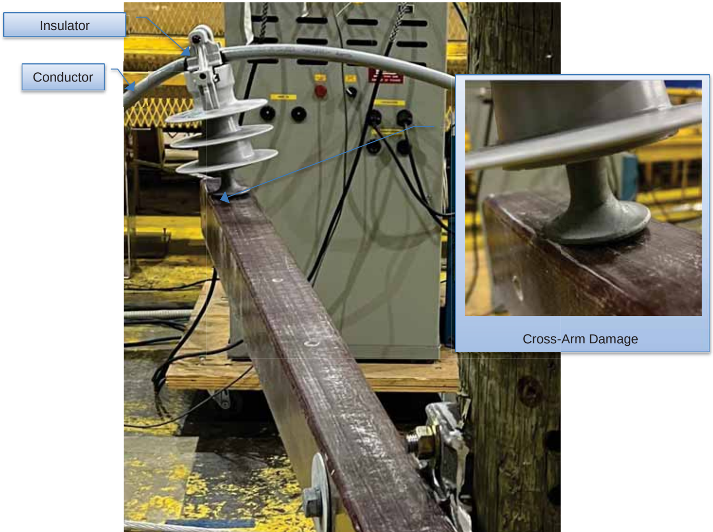
Figure 6-14: Sample 3.2.2 – Insulator and Cross-arm Condition after Test
